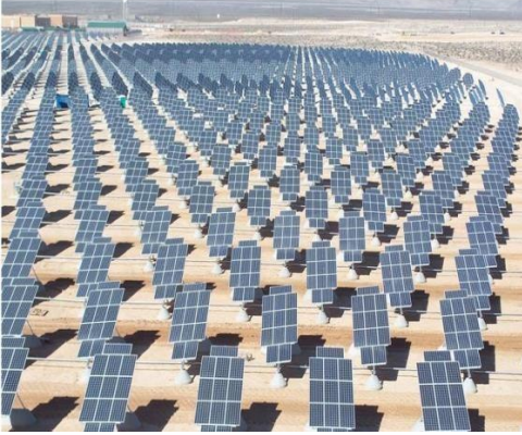
Fig.1. Photo-voltaic (PV) solar farm showing typical arrangement of photovoltaic panels .
